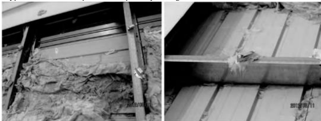
Figure 1. Project damaged by typhoon Haikui in Taiwan [4].
